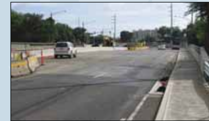
Halawa Stream Bridge Project: New structure opened on Dec 16, 2009. Removal of the detour road and other construction items is anticipated Apr 2010. Completion of landscaping enhancements is anticipated Apr 2011.
